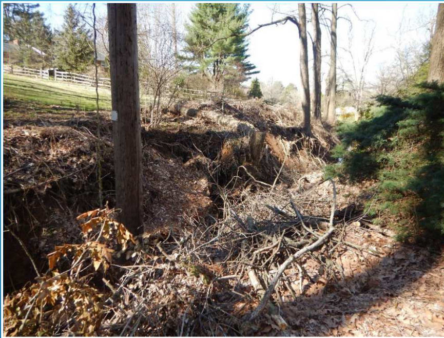
Pole exposed within eroded channel
