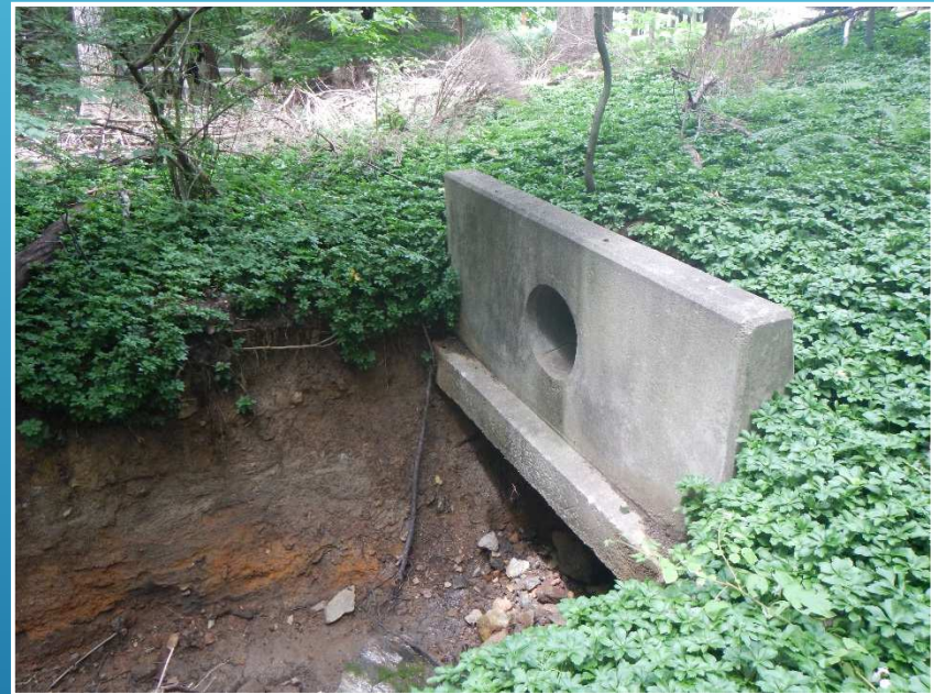
Severe down-cutting at storm drain headwall
