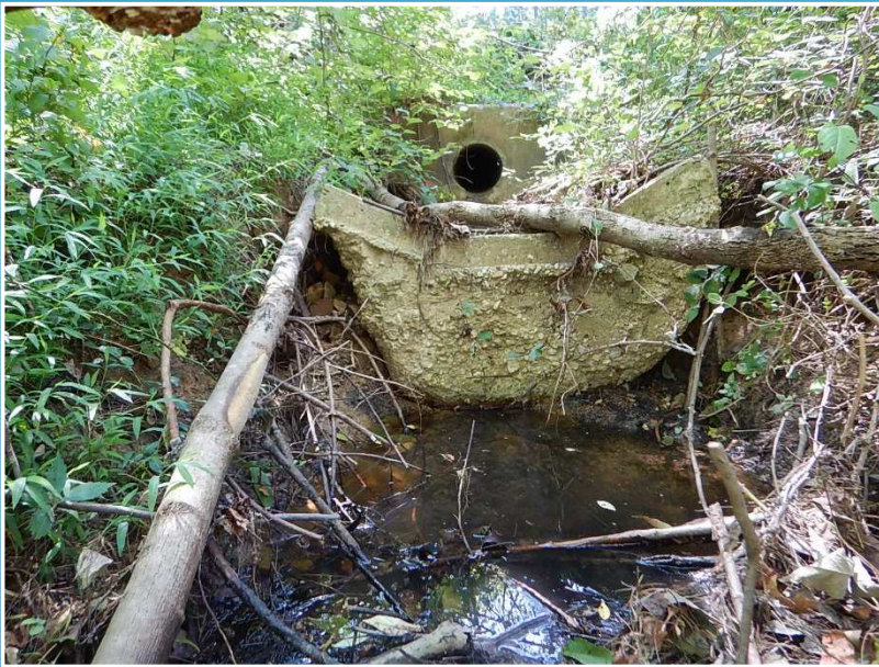
Undercut storm drain outfall at Siesta Garth
