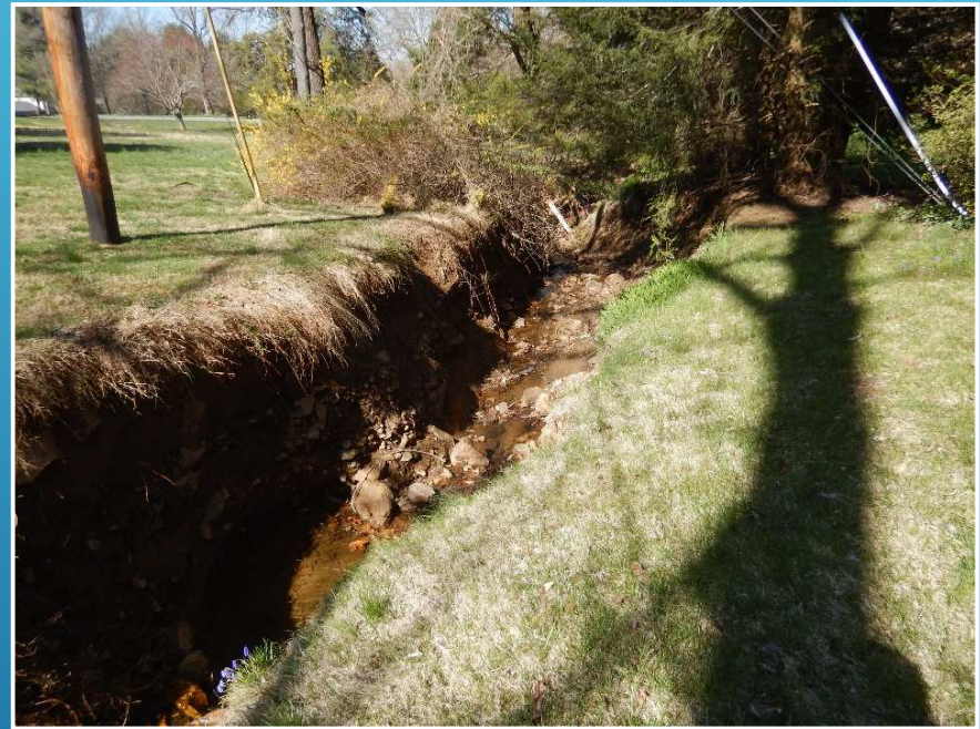
Pole within close proximity of actively eroding channel
