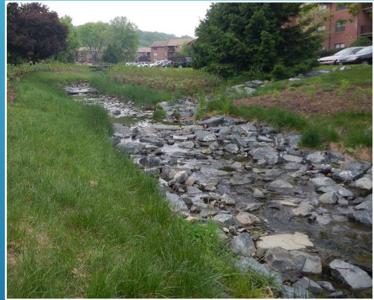
Cascade structures provide stability in steep areas, while also providing habitat for fish and aquatic insects – East Beaverdam II, completed 2014
